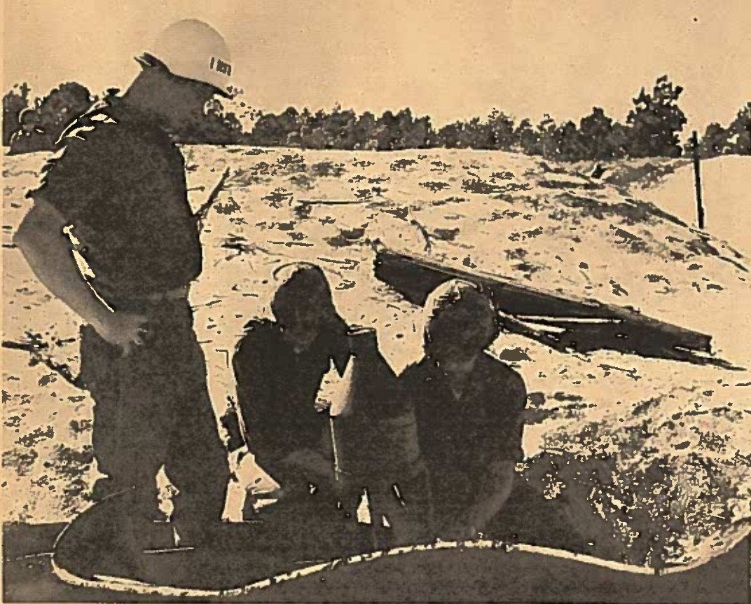
Under the justifiable close observation of their instructor, Constructionman James D. Flory, center, and Lt. Carl E. Christenson keep on as friendly terms as possible with 40 pounds of high explosive as they prepare to cut a steel beam the easy way.
